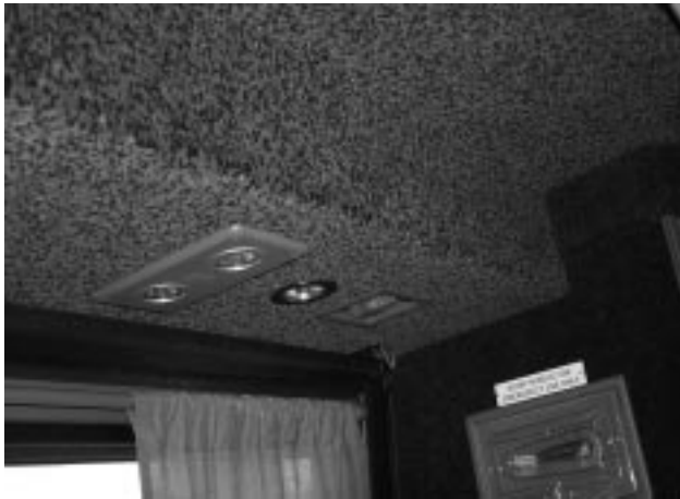
Figure 6b: Parcel rack to restroom flex tube covered by trimmed capping w/ lamp assembly
