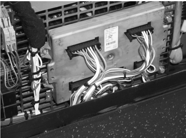
Figure 7: Typical node (this one is located behind the stepwell panel)
