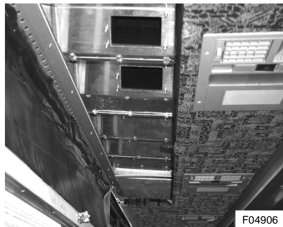
Figure 6: C2045 evaporator blower bank (left-hand parcel rack)
